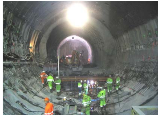
Figure 1: View of the Saint Martin La Porte gallery with the new support system installed.
